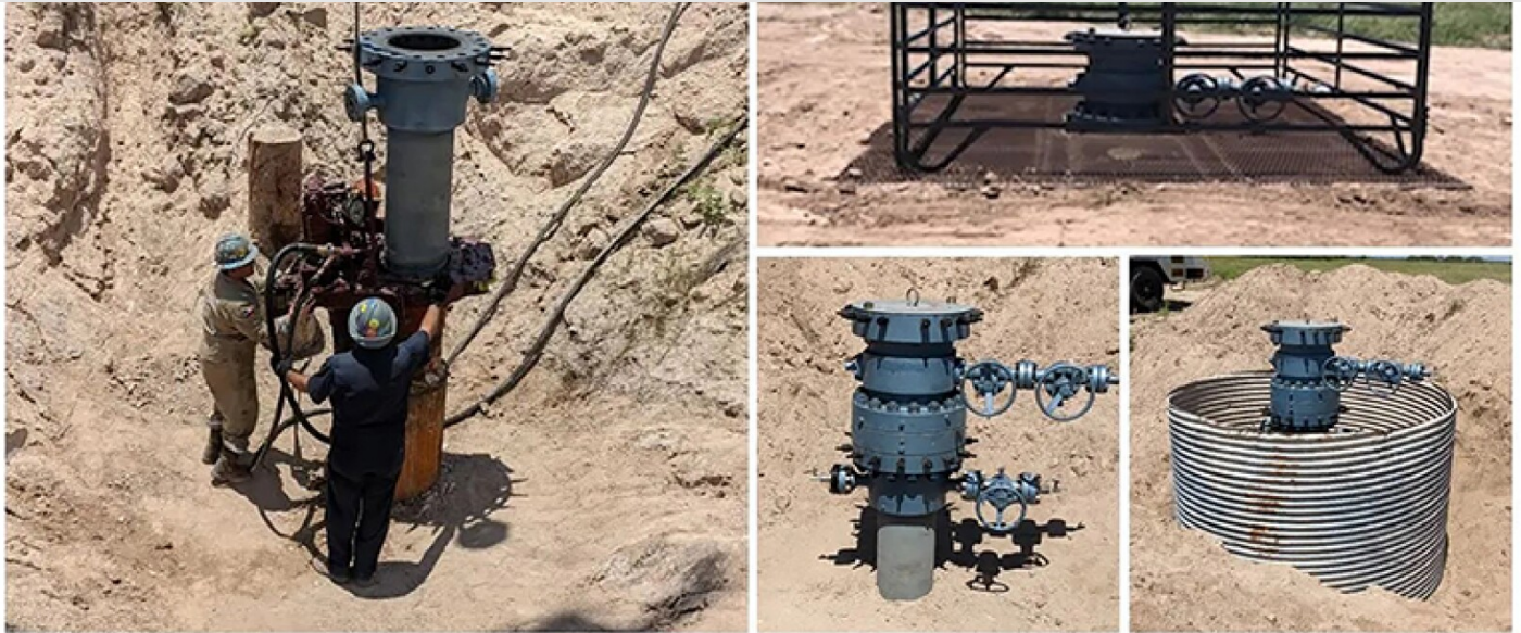
Sage Geosystems installing a new wellhead on a reclaimed Shell well in Starr County, Texas. Source: sagegeosystems.com.
