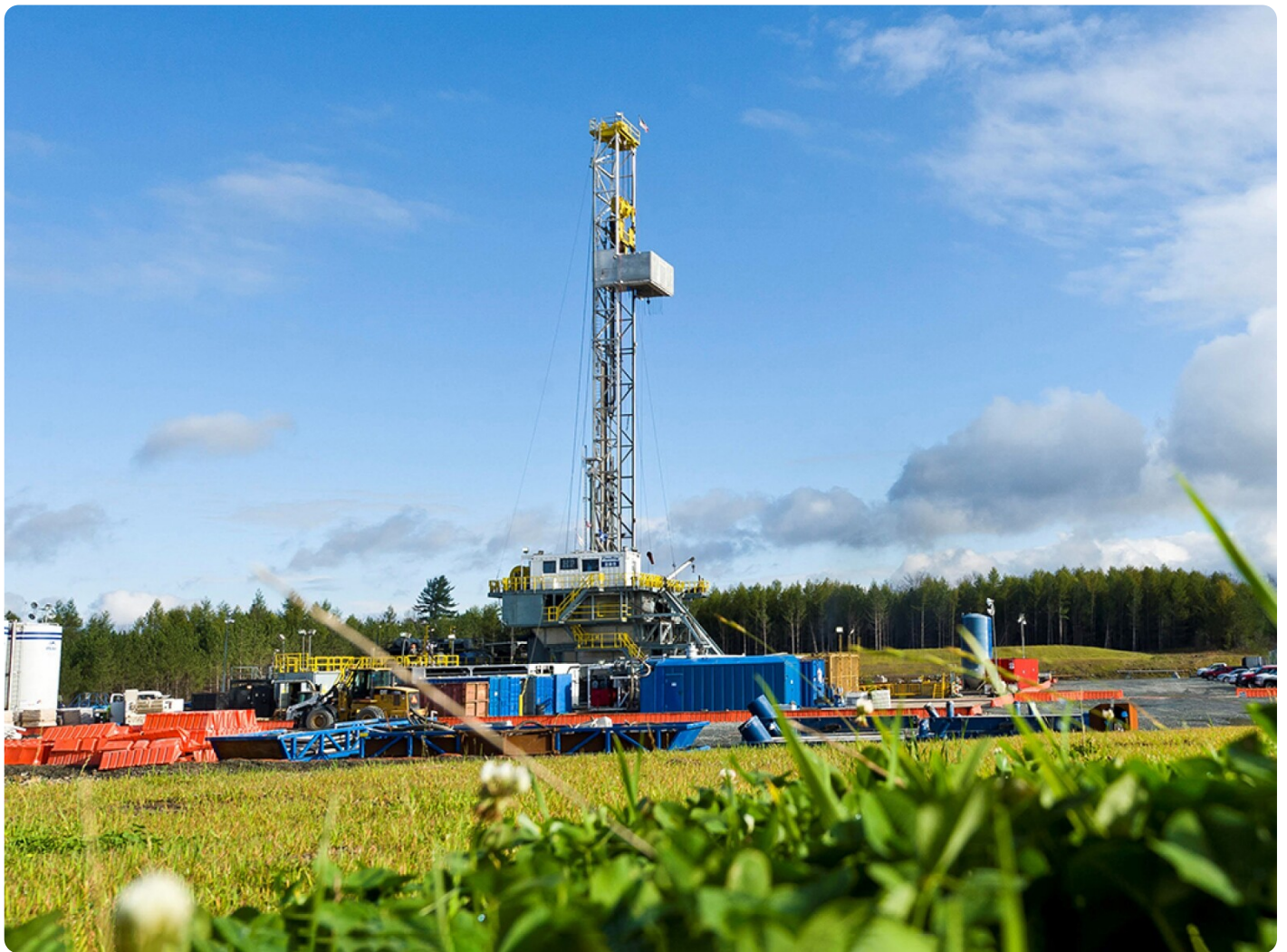
A Nabors rig on location for Sage Geosystems in Starr County, Texas. Source: sagegeosystems.com.
