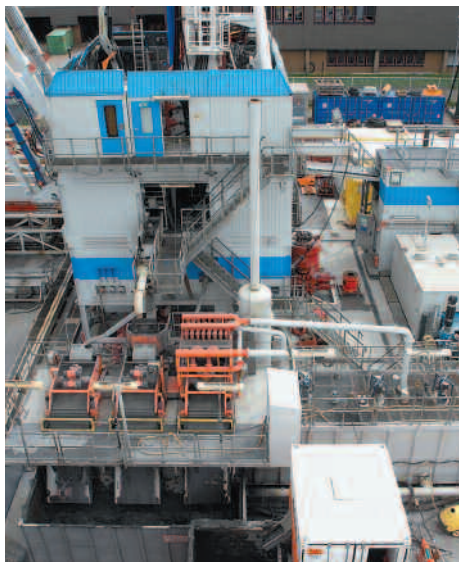
Tank system 240 m 3
