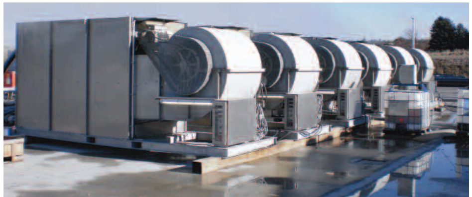
Cooling capacity approx. 21 MW, temperature difference 80 °C to 35 °C
