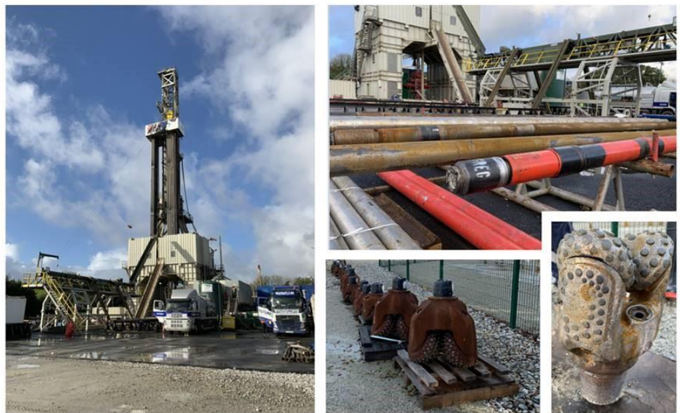
Figure 11: Drilling at Eden Geothermal Limited's site at the Eden Project in Cornwall (part funded by the European Regional Development Fund). Photo credit: Corinna Abesser
