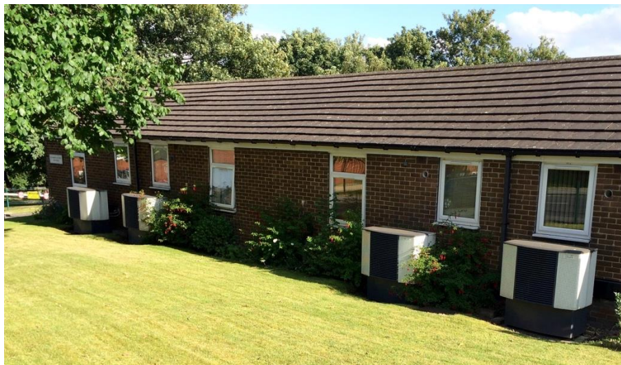
Figure 24. An example of a UK social housing ASHP retrofit installation
