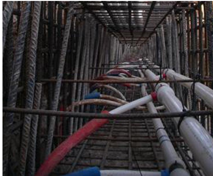
Figure 60. Loop and horizontal tubes connection at the crown beam in Sant Antoni's market
