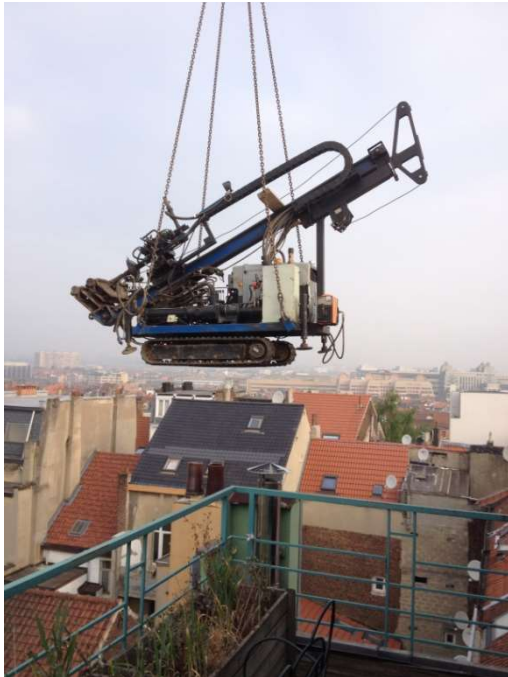
Figure 6: Drilling rig hoisted into place using a mobile crane (photo Geo-Green sprl)
