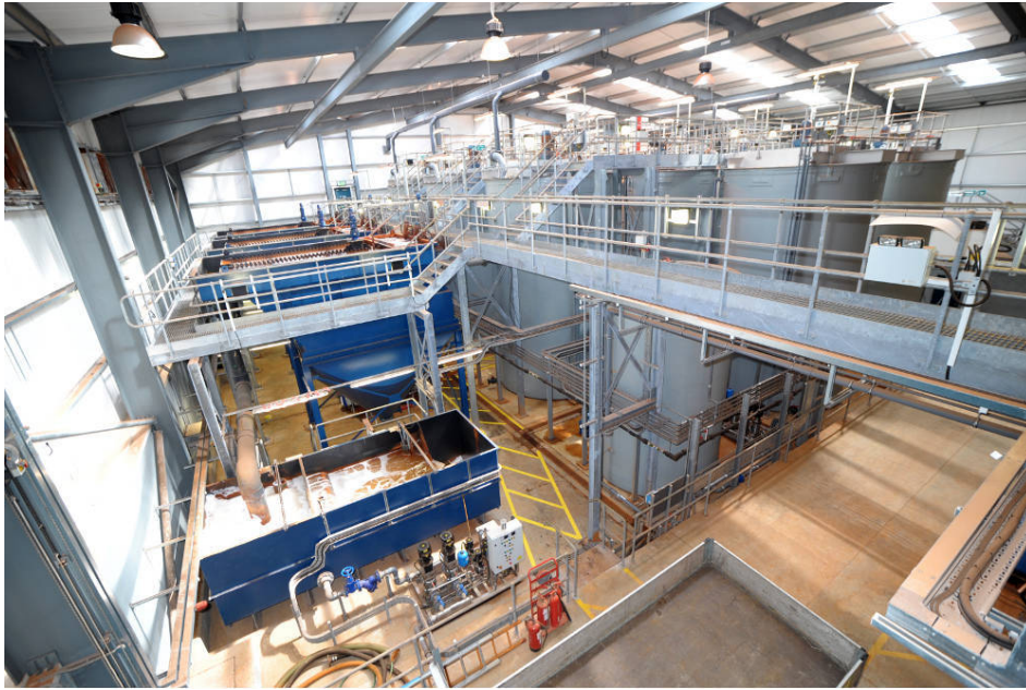
Figure 1.1 The Dawdon mine water treatment scheme that is being developed to supply mine water heating to a new housing complex in the northeast of England. Photo credit: The Coal Authority
